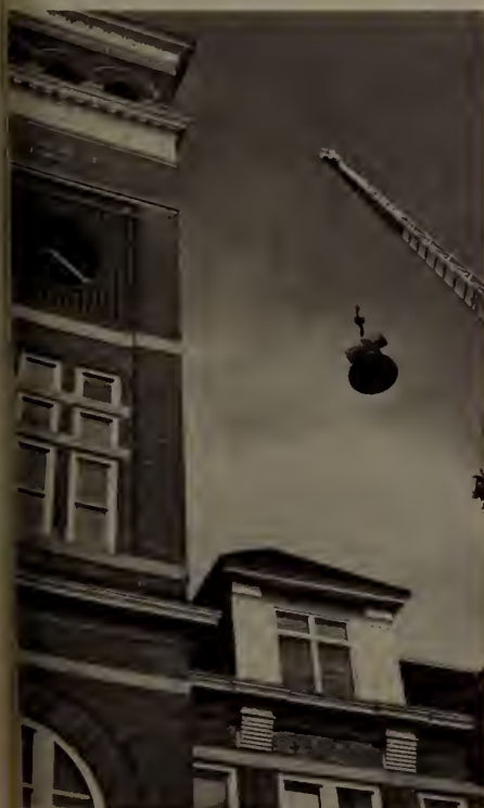
After almost 80 years of timely service atop Tillman, the old bell is lowered from the tower.
